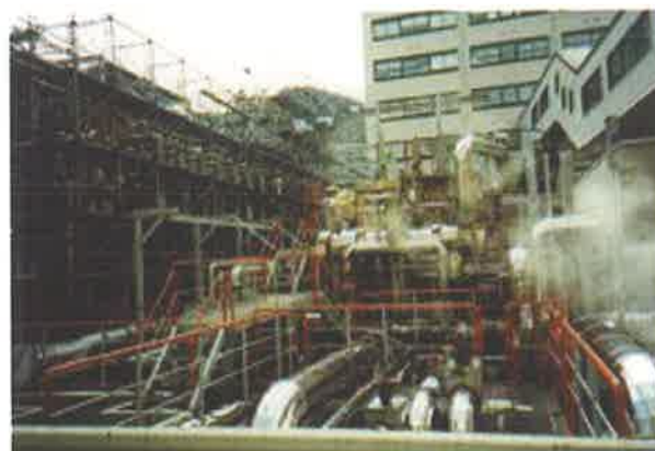
Fig. 3. Operating plant: Ohi, Japan.
